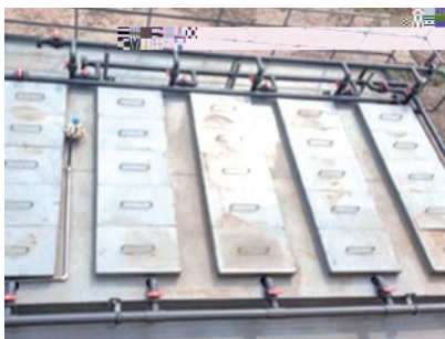
Newly-added advanced processing system
